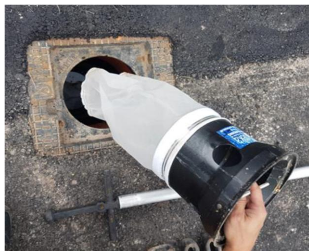
Photo 4: Containment strategy: Drains fitted with filter.
